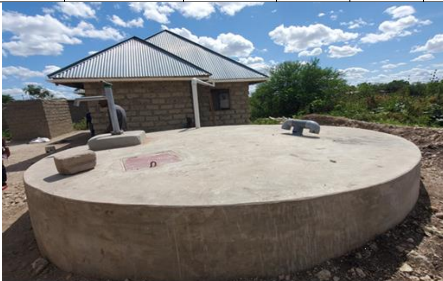
One of the underground rainwater harvest tank handed over to Mazingira and Upendo groups for management and operationalization.
