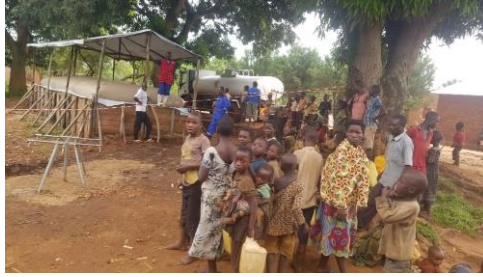
Figure 30 – Installation of a bladder for emergency water supply
