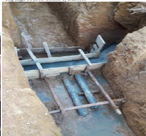
Captage source Chute 1/Basoko
