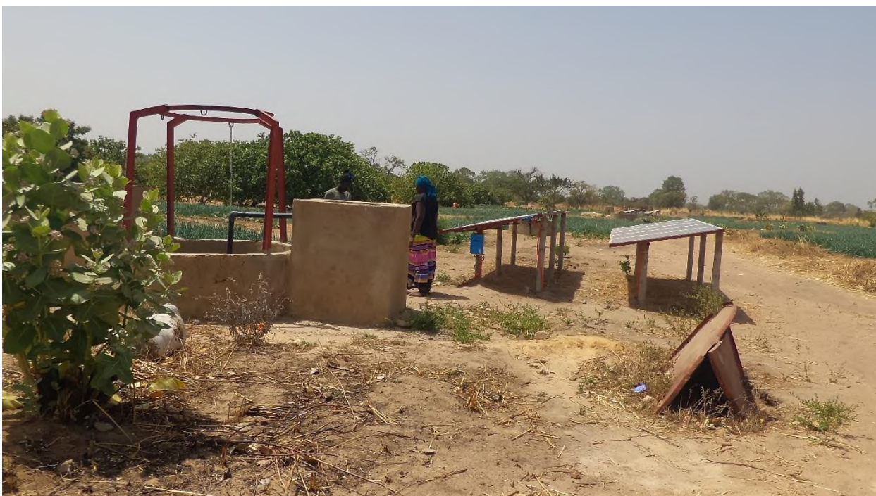
Photo 3: Adaptation - Solar powered water pump and borehole in irrigation perimeter (PARERBA following BARVAFOR)
