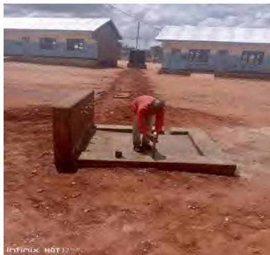
Figure 80: water taps installed at Buguruni primary school – Longido district
